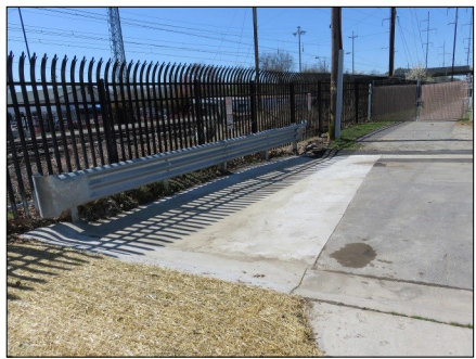
New curb and gutter installed on Old Harmony Road in Robins Green
