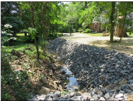
Eroding suburban drainage channel in Chatham stabilized with riprap
