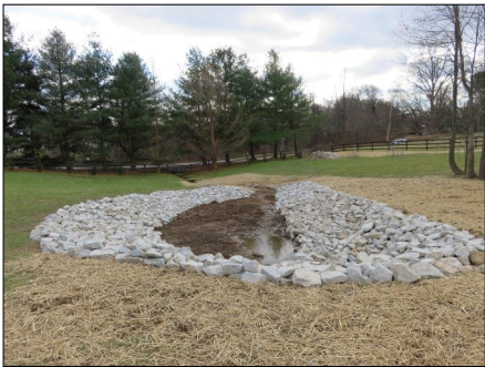
Eroding channel and wet area stabilized in Pierson's Ridge
