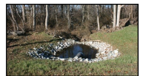
Protected field outlet
