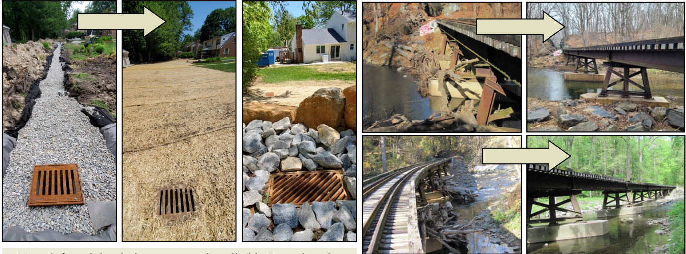
From left to right: drainage system installed in Penarth and a drainage project below a church parking lot off Foulk Road to an adjacent house lot in Chatham.
